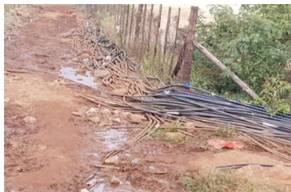
Illegal connections in Raliphaswa village Nzhelele
